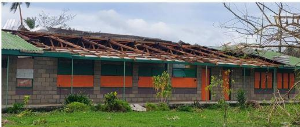
Onesua College Classroom roof destroyed by Cyclone Kevin in March
