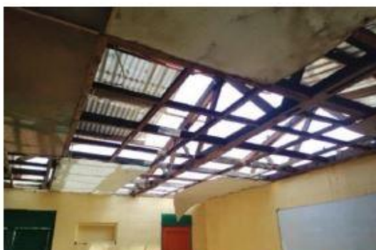
Onesua College – Damage to Junior Science Lab
