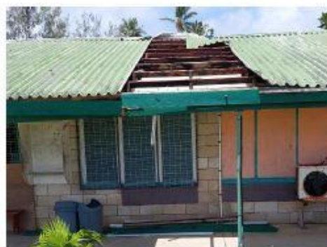
Onesua College - Roof Damage on Computer Lab
