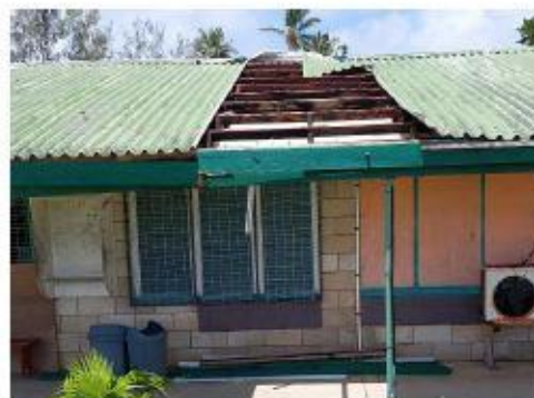
Onesua College - Roof Damage on Computer Lab
