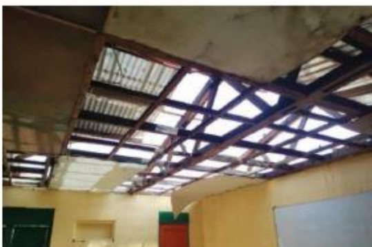
Onesua College – Damage to Junior Science Lab
